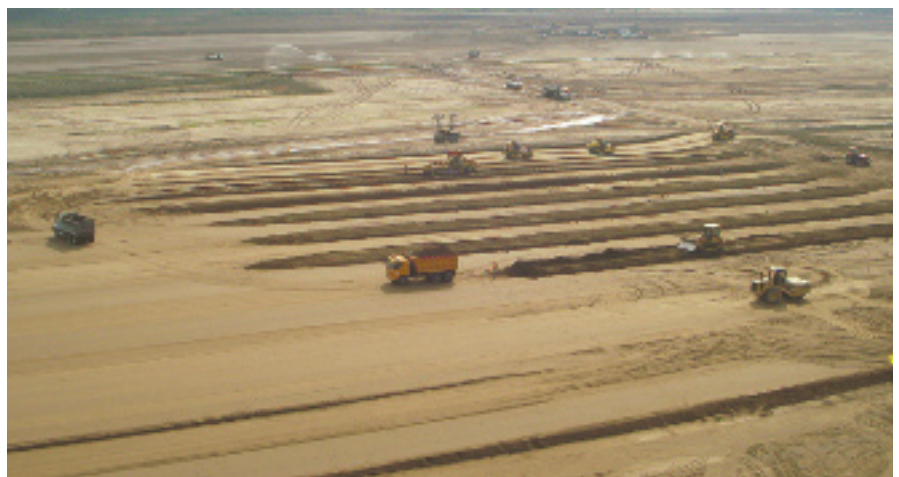
Aerial view of the ground filling and levelling works at the New Quito International Airport construction site
