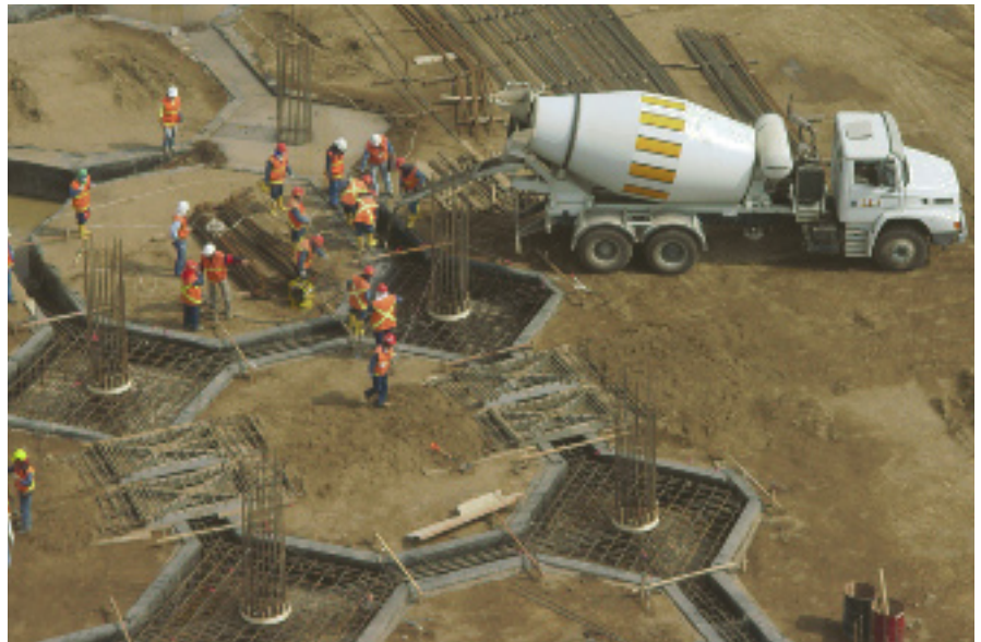
The vertical construction of the New Quito International Airport, currently in progress, began with the laying of the foundations of the passenger bridge
